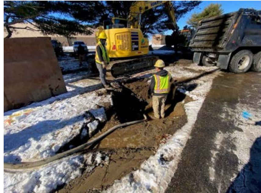
Emergency Water Main Break
